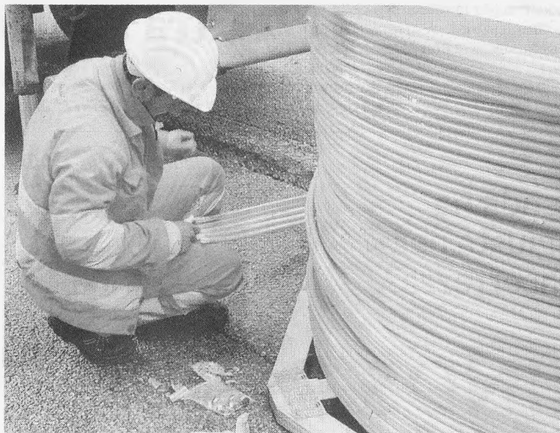
▲ Cavi in fibra
